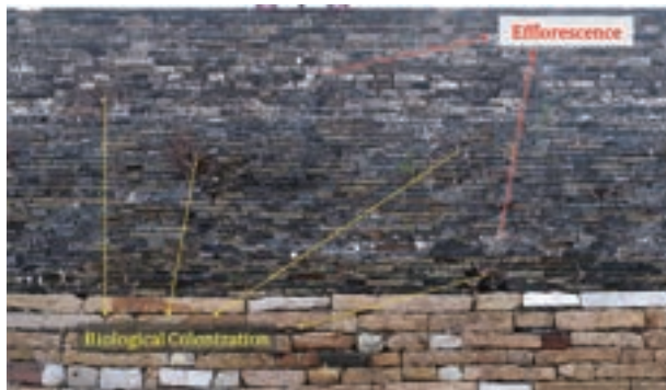
Figure 1. Masonry structures covered by a large area of efflorescence, plant vines and erosion.
