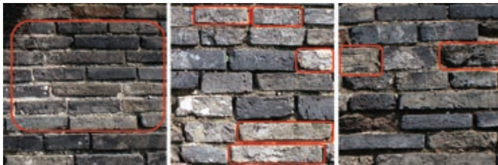
Figure 2. Erosion defect with different damage extent showing different appearance.
