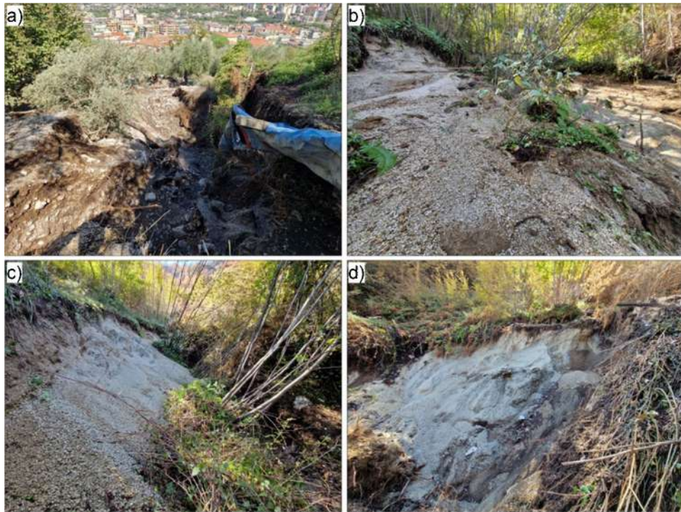
Fig. 9 Ground-based photographs depicting a ) a channel segment in the eastern catchment dominated by erosion; b ), c ), d ) scarps of lateral landslides
