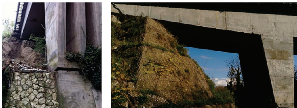
Fig. 4. The landslide of the slope in 2015 and the armed lands behind the pier.
