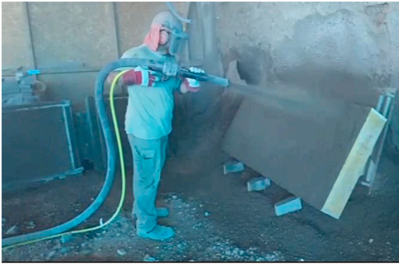
Fig. 2. Shot-earth technique. The air stream is projected at a high velocity onto the receiving surface, representing the formwork panel.
