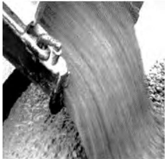
Fig. 1 Getto di calcestruzzo autocompattante mediante pompa / Jet of self compacting concrete by pump
