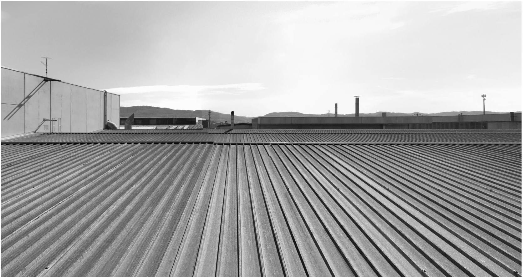
Fig. 3 - Sheet metalfields. Industrial countryside in Bagnoli di Sopra (PD), I (photo by R. Ghirardi, 2019).
