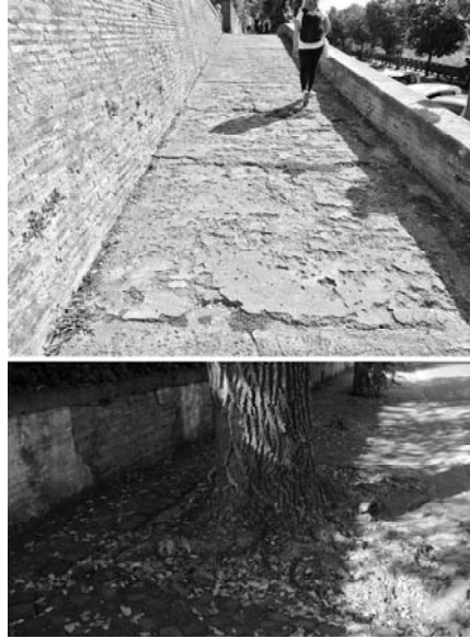
Fig. 5 - Examples of road pavement failure
