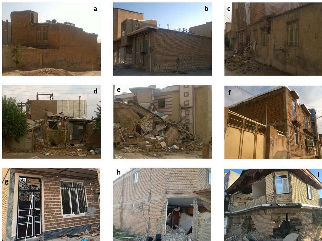
FIGURE 1 | Damaged Sarpol-e-zahab masonry building samples (a) URM D1, (b) URM D2, (c) URM D3, (d) URM D4, (e) URM D5, (f) CM D1, (g) CM D2, (h) CM D3, and (i) CM D4 (original).
