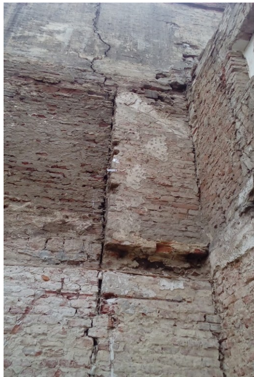
Fig.4 Cracks on the longitudinal central wall
