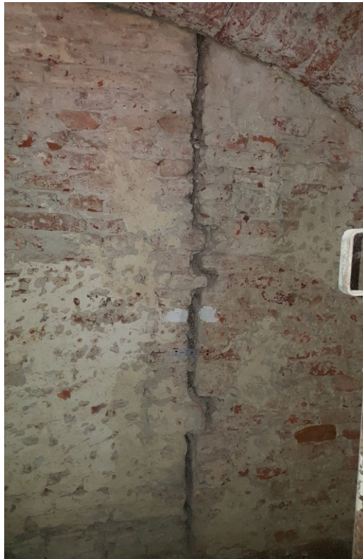
Fig.3 Cracks at the first floor
