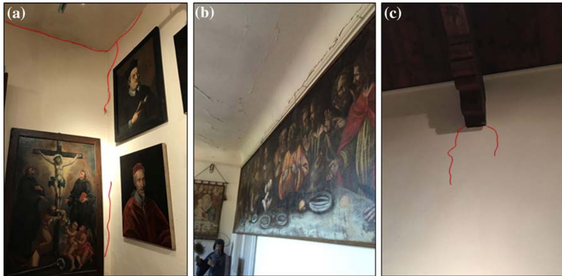
Fig. 4 Some damages in the camorcanna and in the connection between transversal walls (a), only in the camorcanna (b) and in the connection between wooden beams and walls of the facades (c)
