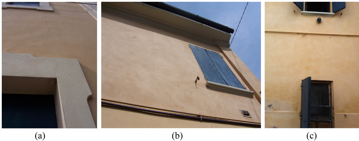
Fig. 11. Some spandrels damaged after earthquake: agreement between real collapse mechanisms and numerical ones (see Fig. 10).
