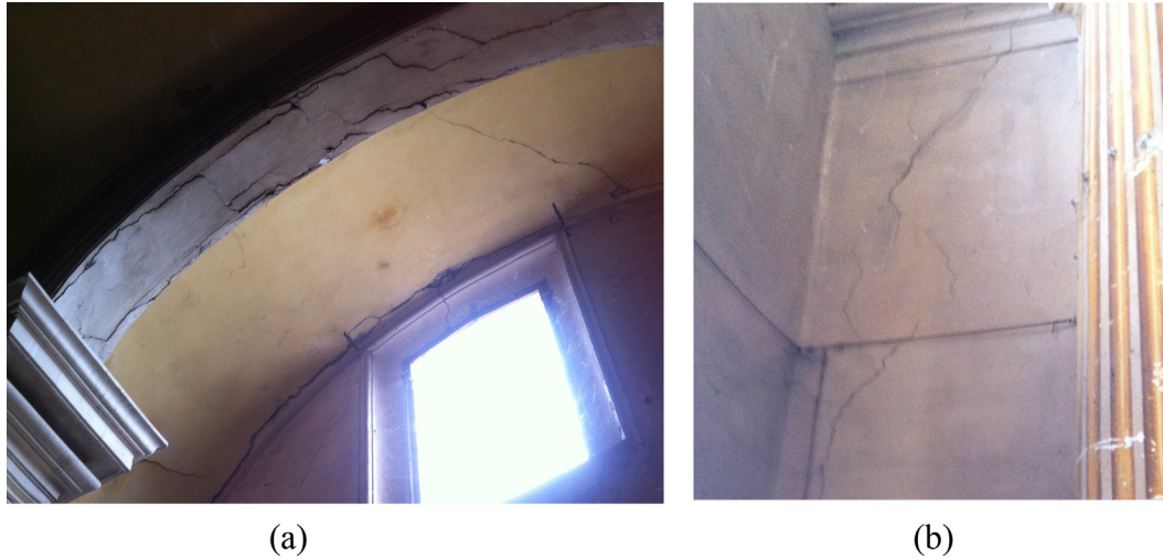
Fig. 5. Cracks into arch and vault (a) and pier diagonal cracks (b) in the oratory.
