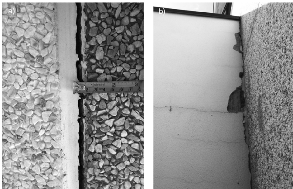
Fig. 32. Column-panel detachment (a) and vertical crack due to hammering effect among adjacent buildings (b). Distacco colonna-pannello (a) e fessurazione verticale dovuta a martellamento tra edifici adiacenti (b).
