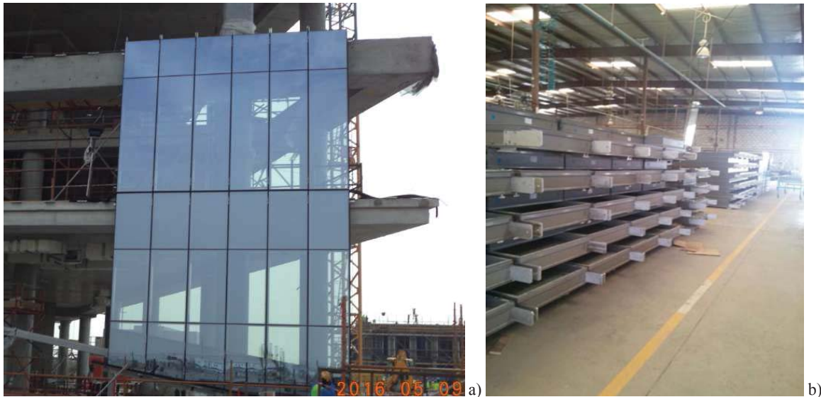
Figure 5. Mock up of 12 panels (a) and production of unitized panels (b) for the NPP 0064 Mwani building
