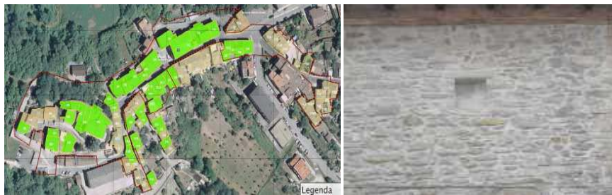
Figure 24 (a) Investigated units (b) Typical masonry wall of the Arsita built-up (see online version for colours)
