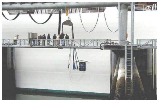
Fig. 3 Cold ironing arrangement in Juneau (Alaska)-2-
