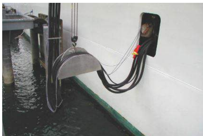
Fig. 2 Cold ironing arrangement in Juneau (Alaska)-1-
