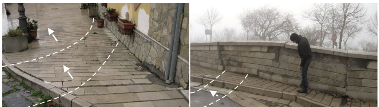
Fig. 4 Effects of ongoing slope movements
