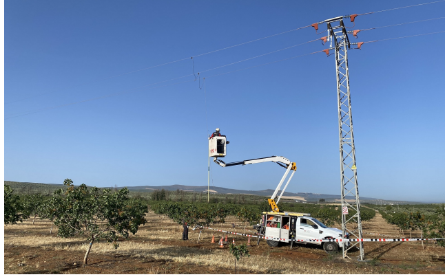
Figure 1: Human operator on elevated working platform grounding the three phases of a power line section close to the ATLAS Flight Center before conducting a maintenance task.
