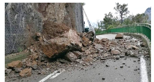
Fig.5 – Boulders coming from a rockfall located near a bend of the Amalfitana state road.
