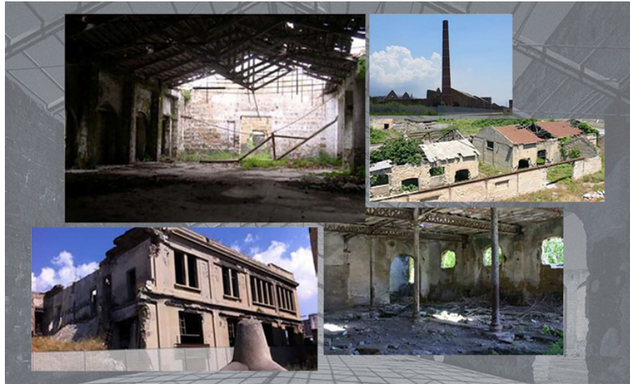
Fig. 4. State of some pavilions of the industrial complex of the former Corradini foundry in Naples (image: M. Falcone, G. Angrisani).
