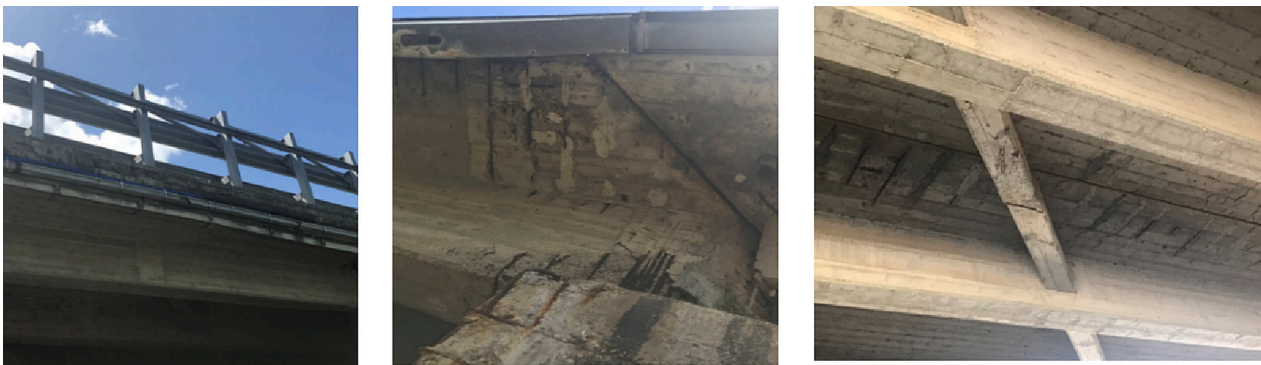
Fig. 15. Photographs taken with the Drone.
