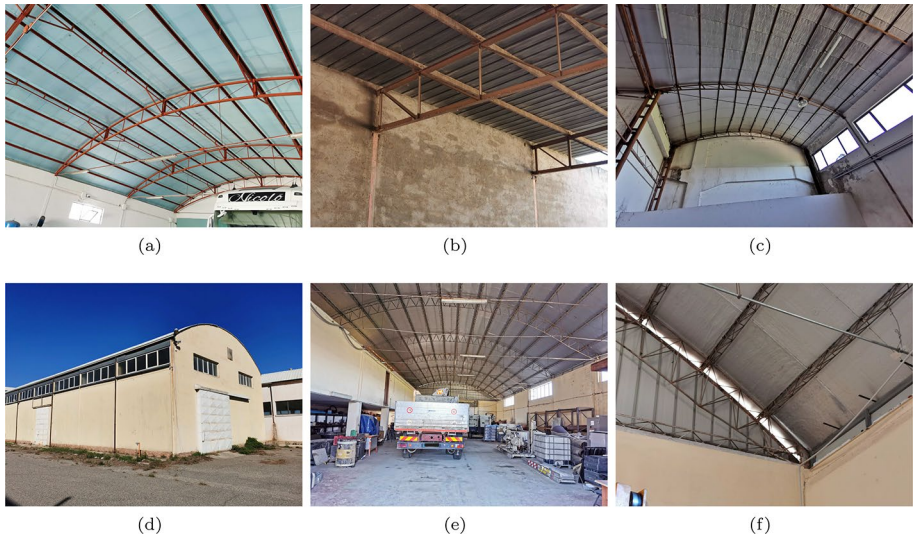
Fig. 5 Some pictures of the industrial structures in the area under consideration. It is possible to observe the geometry of the curved roof truss (a, c, e), the connection between truss and columns (b, f) and a view from the outside (d)
