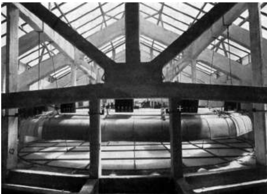
Figure 10. Martinotti, Detail of the fluorescent lighting installation. Pinacoteca di Brera, Milan. [Source: Wittgens, "La ricostruzione," 364, fig. 8]
