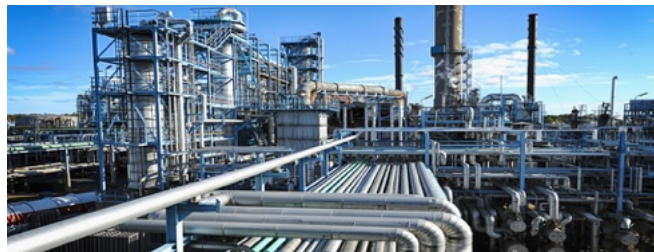
Fig. 1: Pipe racks structures
