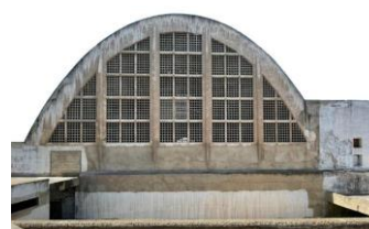
Figure 21. Decays on South Facade
