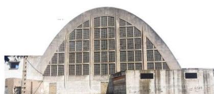
Figure 20. Decays on North Facade
