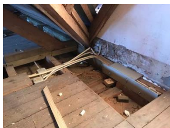
Figure 8. Repair of connections between roof structure with floor beams (credits: Aníbal Costa)
