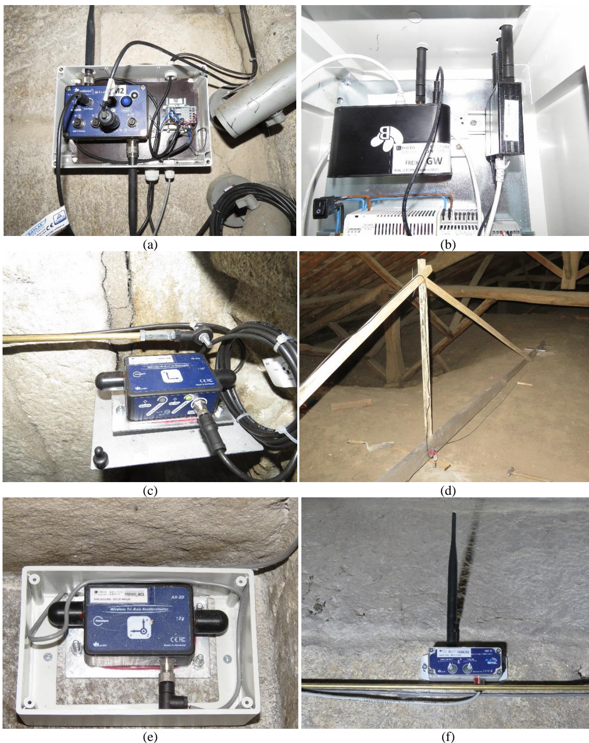
Figure 5. Monitoring system installed: (a) acquisition module M2; (b) gateway; (c) tiltmeter (CL2) and extremity of crackmeter FS3; (d) crackmeter FS7 installed on the extrados of the vault; (e) accelerometer (AC1); (f) temperature sensor TH1 and the extension rod of the crackmeter FS2 [source: authors].
