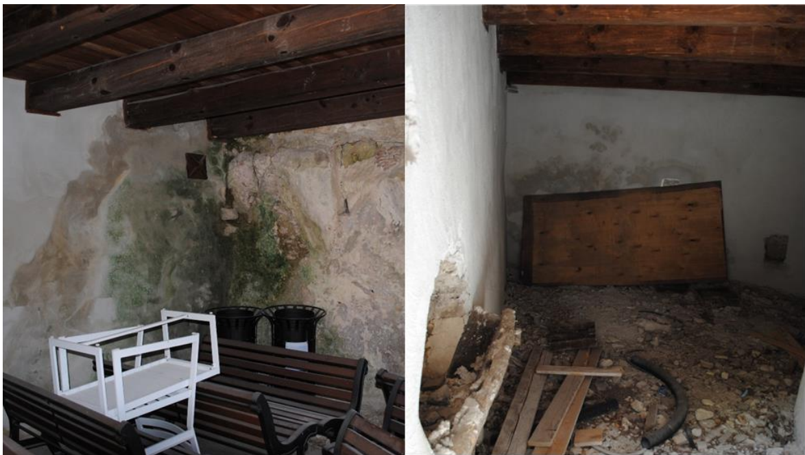
Figure 5. Degradation of the interior.
