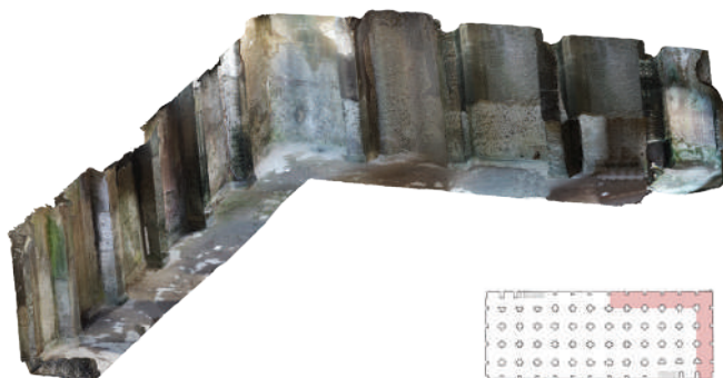
Figure 4. Axonometric view as a result of the photogrammetric process, with the study area highlighted in color.
