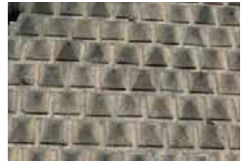
Figure 10 : Detail of the façade of the Church of Gesù Nuovo (photo by author)
